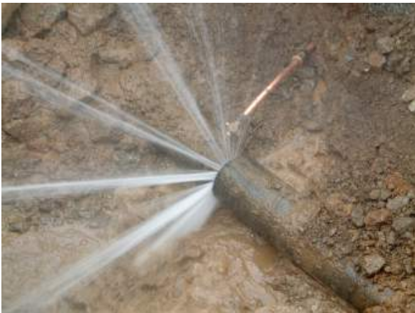
Fig. 1: A damaged pipeline
